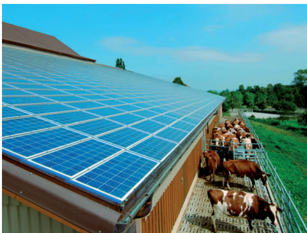
Photovoltaikanlage Aeberhard in Barberêche, naturemade star
